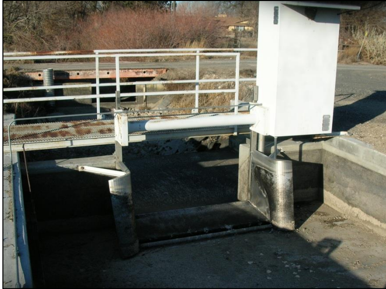
Gate for Spillway No. 4
