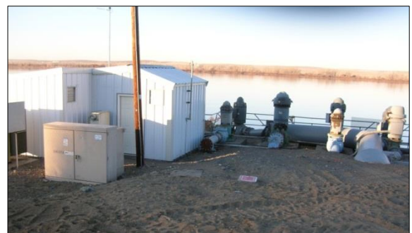
Irrigon Pump Station (IPS)
