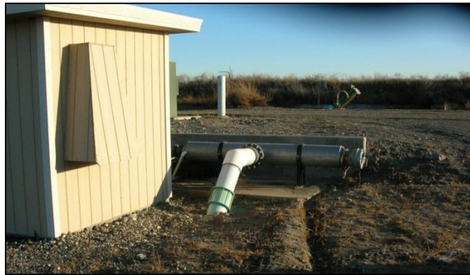
RL2 Booster Station
