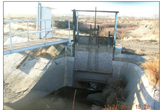
Gate for Spillway No. 3 at I-84 Siphon
